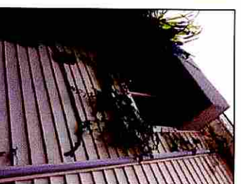
NON HISTORIC NORTH WINDOW WINDOWS TO BE COME EXTERIOR DOOR AT GRILLING PORCH
