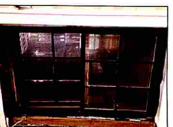
GROUND FLOOR WINDOWS EXAMPLE CONDITION OF GROUND FLOOR WINDOWS TOP SASH TRAIL MISSING
