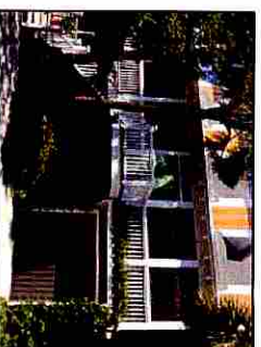
2216 TON RAILING AND SCREEN DOOR WITH SIDE STAIRCASE NARROW FRENCH DOORS ONTO PORCH
