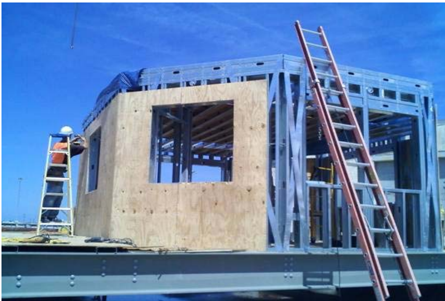
Photo caption: With new framing completed on the new bridge’s control house, construction begins on closing in the building’s walls.
